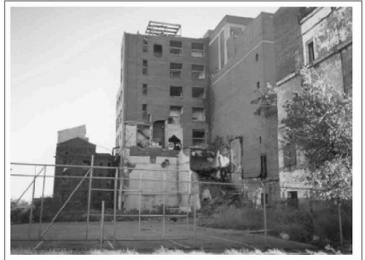
FIGURE 1 I took this picture because it is an abandoned building, and nobody pays it attention. It's somewhere that I have visited, and I've seen the inside. I knew there was more to it than just what is on the outside. I noticed the flooding in the basement. I noticed the holes in the ceilings and floors. Also, I noticed rusty elevator shafts. One whole floor had metal rails all across it. The entire floor was nothing but metal rails. Kids go there because it's fun, and it's a place to get away from adults nagging. It was once a nice building, and now it is decayed. I think it's a bad idea for kids to go there, but it's fun.
